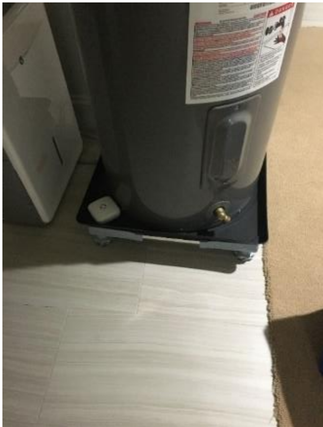
Figure 1: electric water heater with a water alarm in the catch pan
