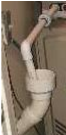
Figure 3: building drain serving a single AC unit
