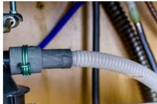
Figure 7: correct drain (silicone rubber)
