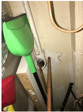
Figure 4: building drain serving two (2) AC systems
