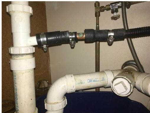
Figure 6: leak-prone drain (hardened black rubber)
